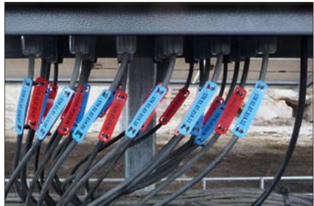
TAGPU for clear identification of multiple strings.
